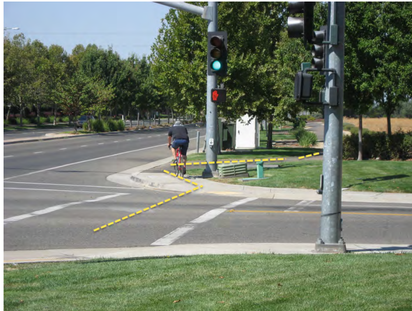
Current Situation – The existing curb cut requires several sharp turns around curbs, light standards and utility equipment. This configuration is very difficult to navigate and nearly impossible with a child carrier trailer.
